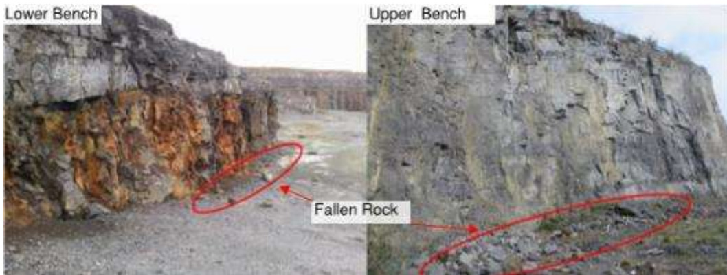
Figure 3.5: Face instability on the lower and upper bench
